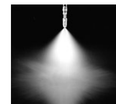
The fine water mist from the nozzles.
